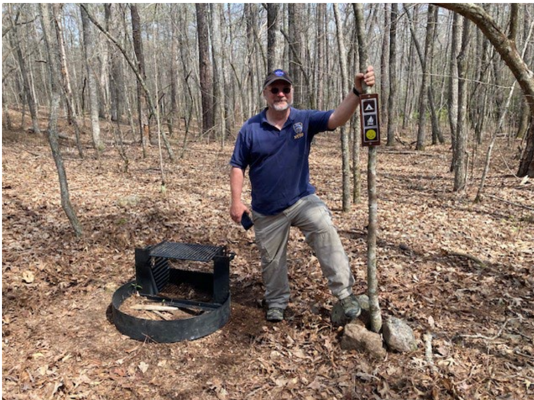
Eddie Hall on March 20, 2024 helping install fire ring and install signs and post.
